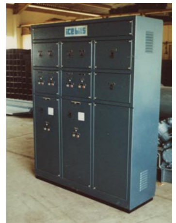
Electric Switch Board central control of all electric operations in the plant
