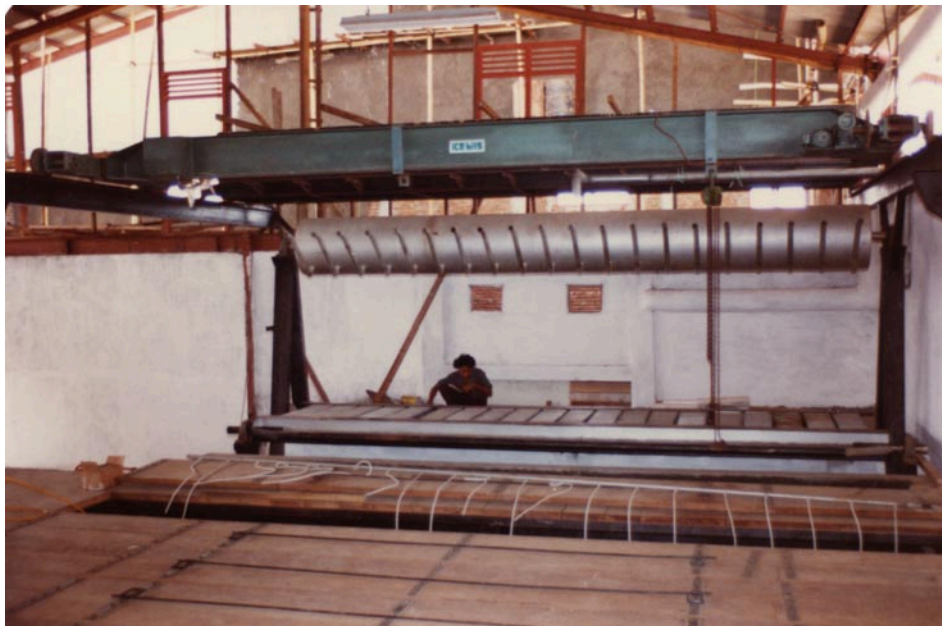
The picture above shows an Overhead Gantry Crane and an Ice Can Filler to refill twenty (20) square 25 kg ice cans at a time, for a 50 mTon/24h plant built by IceBits in Singapore in the early eighties and delivered to Pekalongan on Central Java, Indonesia.
